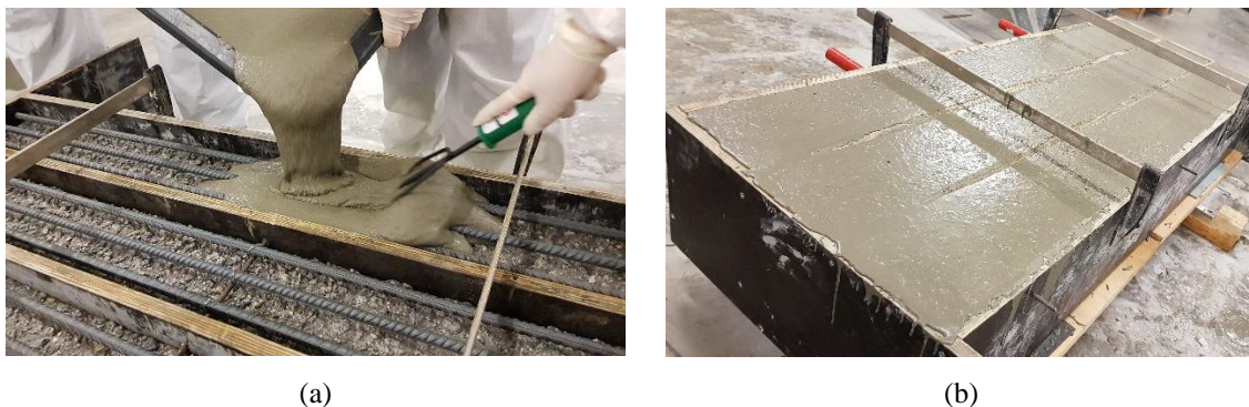
Figure 68. Casting of the RU layer in Series VB: (a) pouring the UHPFRC; (b) final aspect.
