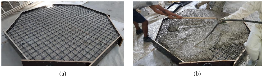
Figure 89. The casting of RC overlay of the PC-RC specimen: (a) reinforcement layout; and (b) concrete placement.
