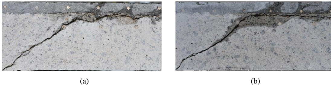
Figure 93. Typical detail of the critical shear crack and NIC in slab PE-RU1: (a) South and (b) East.
