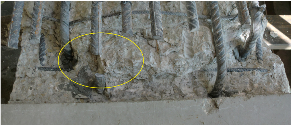
Figure 5.30: Rupture in the reinforcement (beam III.C)
