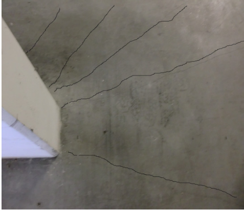
Figure 1.1: Cracking pattern around the columns (Building Visconde de Alvalade )
