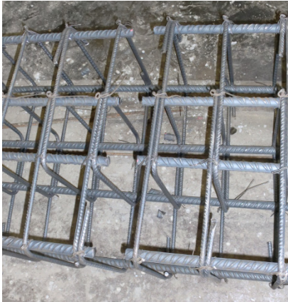
Figure 4.7: Interrupted longitudinal reinforcement (substrate)
