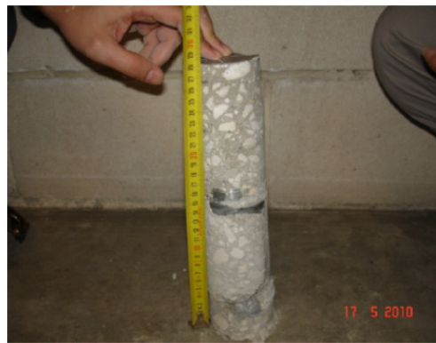
Figure 2.6: Core extracted from the slab in -2 level (while the thickness is 0,28m, the concrete cover of the top reinforcement measures 0,1m)
