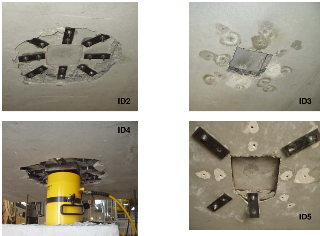
Figure 5 : Bottom surfaces of Models ID2 to ID5 after punching failure
